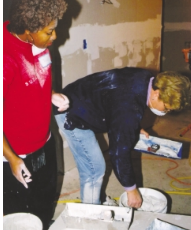
Curtese Howard and Lauren Scanlon work on a drywall project at a Habitat for Humanity house. Students volunteered at several locations on the Big Event day.
